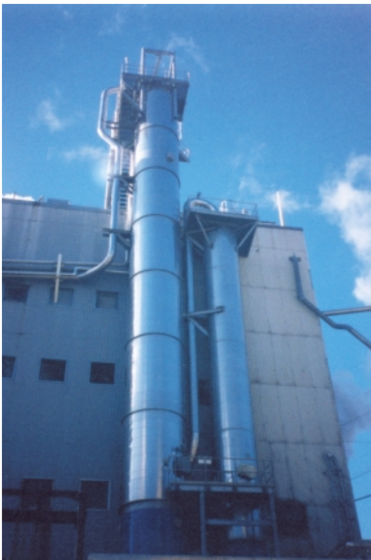
Lincoln's new No.1 and No.2 oxygen reactors
