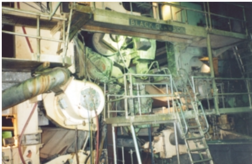
A view of the old Vertiformer—to be replaced with a Valmet Optiformer—on PM 11
