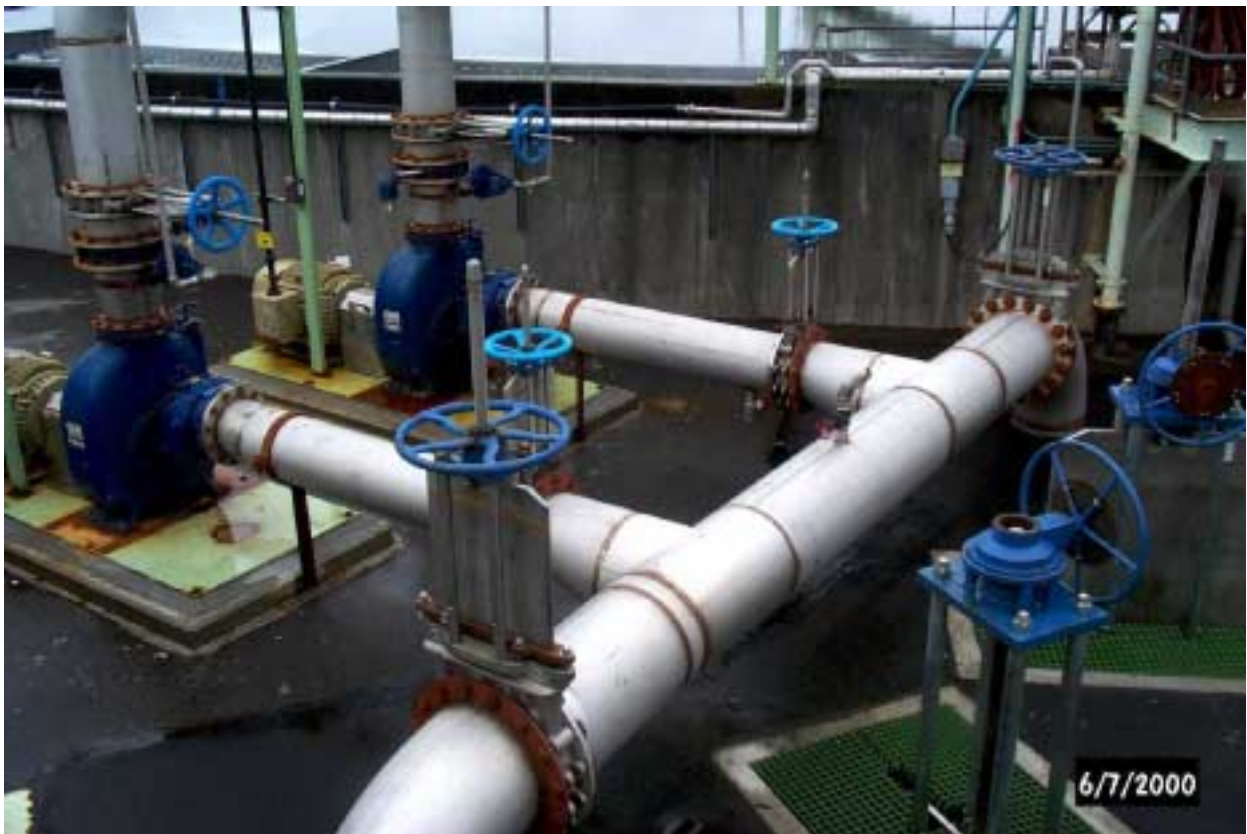
Figure 4. DCD effluent pump installation.
