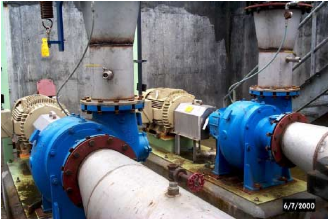
Figure 3. DCD RAS pump installation.
