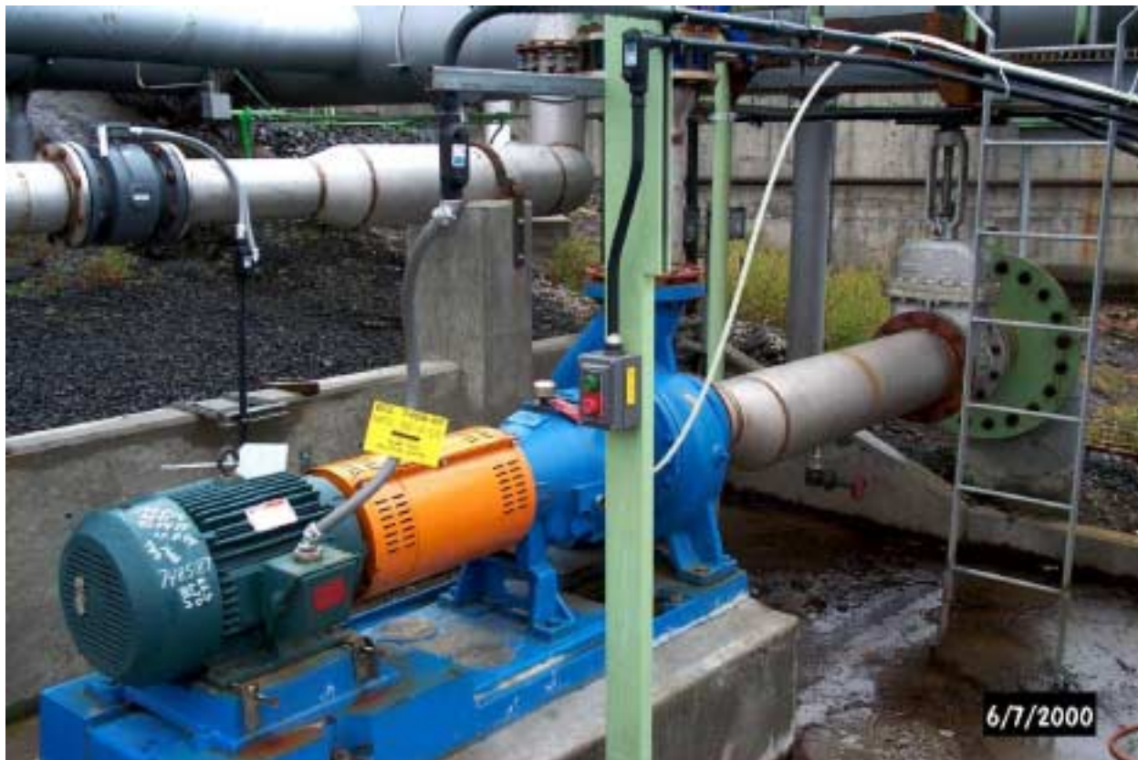
Figure 5. Dilution pump installation.
