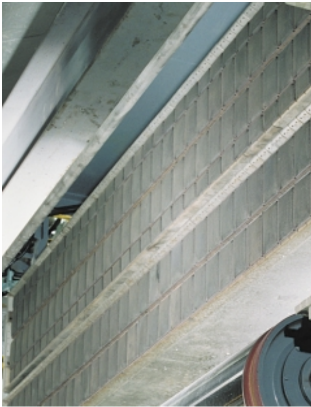
6. Gas drying frames are mounted opposite each other
