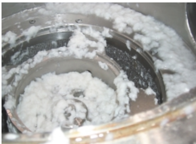
6. Secondary slotted screen showing some PSA. Note that most are fiber flock with no PSA content.
