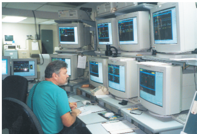
The control room for the No. 4 paper machine
