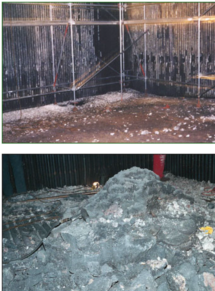
Figure 4. Examples of a recovery boiler where the smelt bed has been nearly completely burned-out and a boiler where little effort was made to remove the bed before shut-down.
