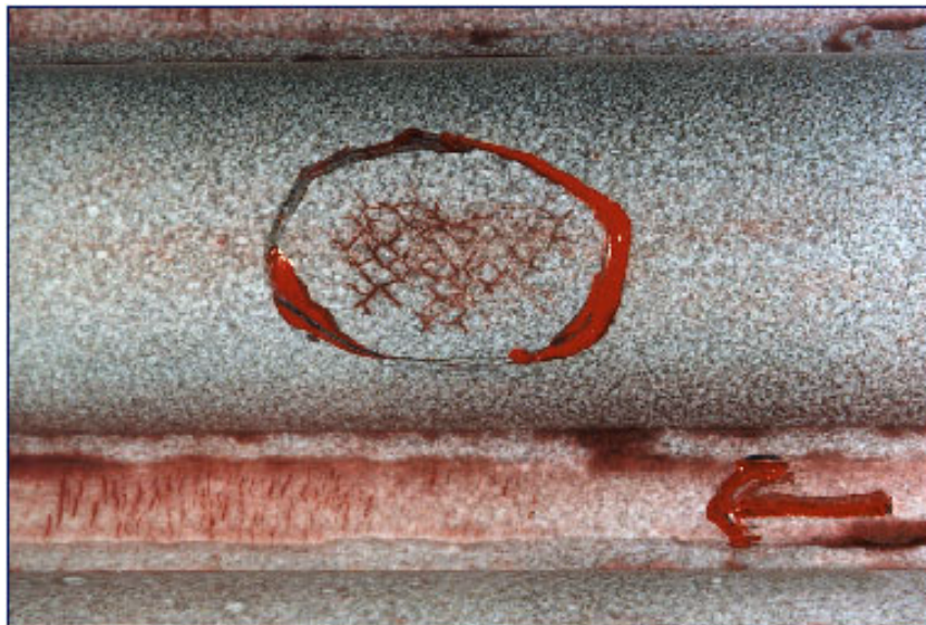
Figure 3. The craze or interconnected cracking found on some tubes suggests that both axial and tangential stresses are tensile.
