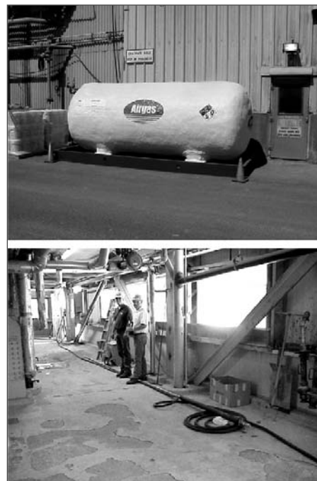
5. Liquid CO 2 storage tank and lance.
