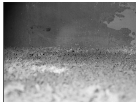
3. Black deposit that accumulated on the heat exchanger's surface.
