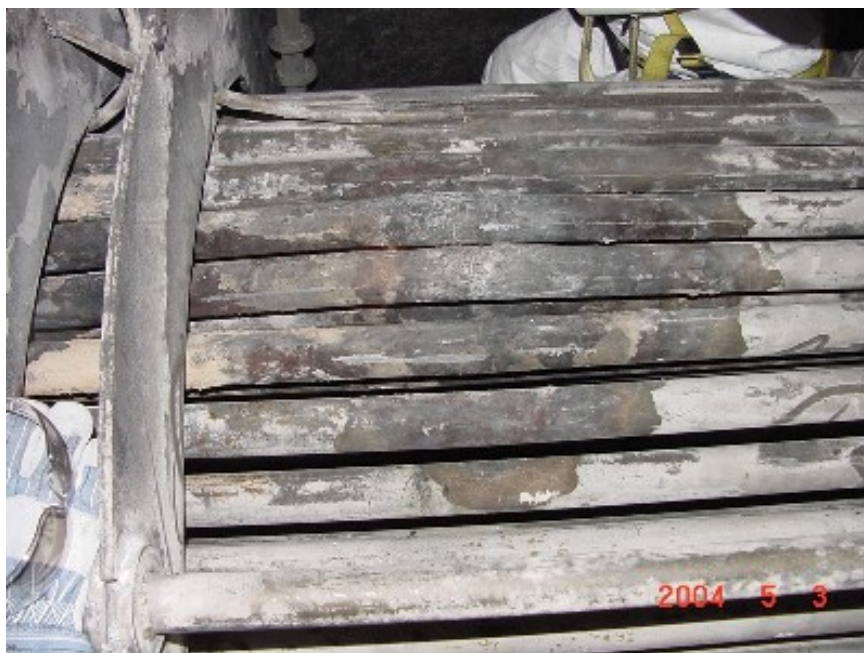
Figure 11. Photo of the heater tube bundle from which the tubes in the previous figure were taken. The two damaged areas of the tubes are slightly above center in the picture.
