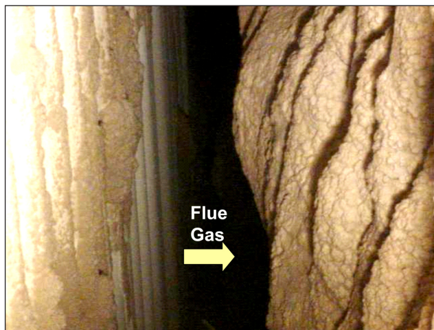
1. Heavy deposit buildup at the generating bank inlet of recovery boiler A (RB-A).
