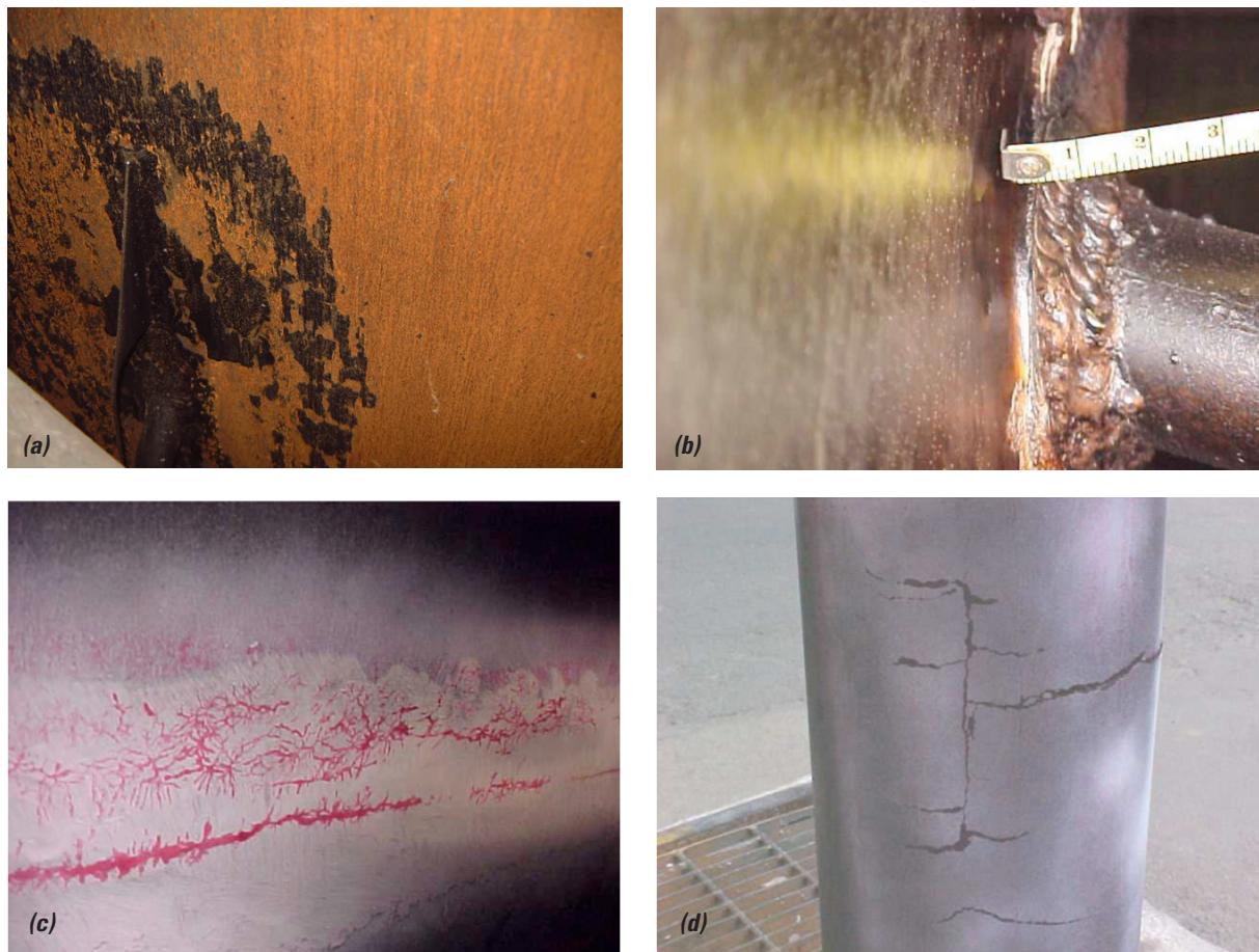
5. Corrosion aspects observed in digester 1: (a) and (b) shell corrosion thinning, (c) stress corrosion cracking (SCC) on the stainless clad plates of the upper zone, (d) central pipe destroyed by SCC.
