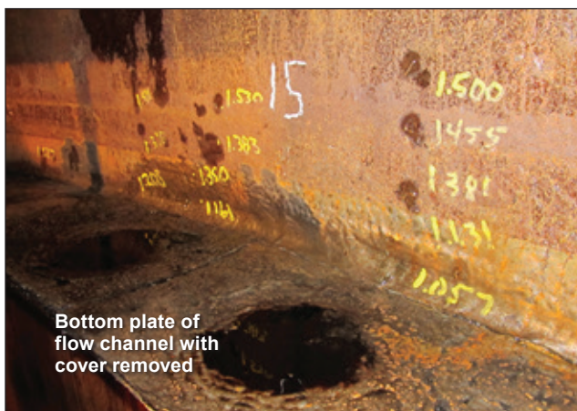
5. Erosion-corrosion damage to the digester shell and bottom of the flow channel.
