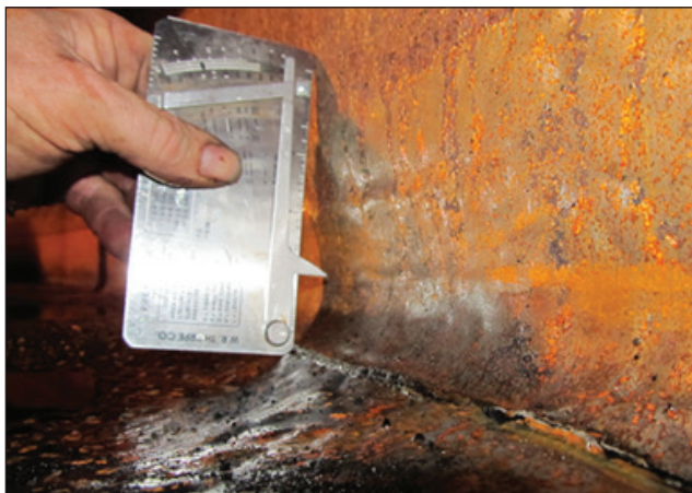
4. Inside the lower extraction flow channel with cover removed for access.
