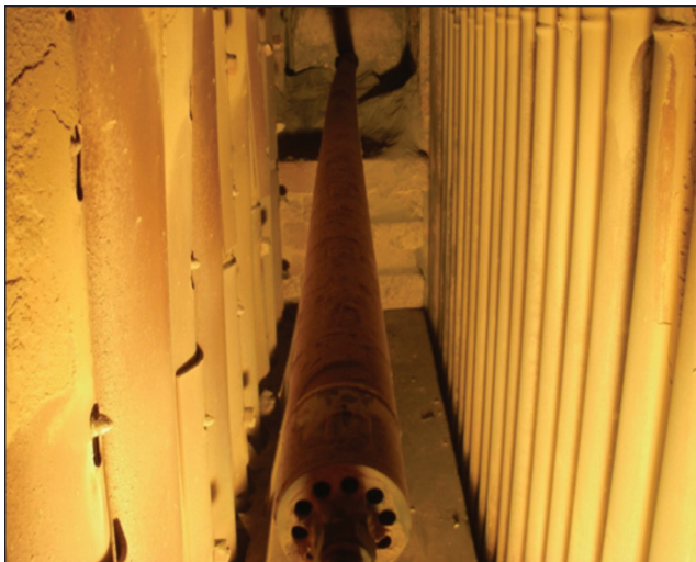
13. Photo of the corrosion probe in the Gadsden power boiler just prior to its removal (photo courtesy of Billy Zemo, Southern Company).
