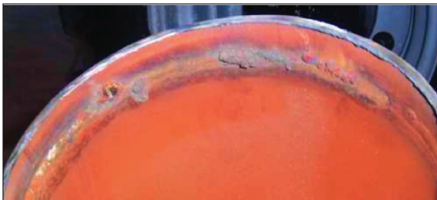
21. White water piping: Rust mounds at corrosion sites at a circumferential weld in a hot water pipe.
