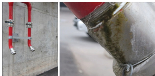
6. Growth of green algae at a water leak where a fire water outlet nozzle cap was screwed to a fire water pipe.
