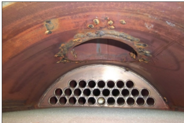
12. Heat exchanger 2: Pass 4 tube sheet beside the cooling water discharge nozzle.
