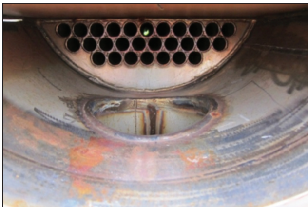
13. Heat exchanger 2: Clean surfaces of the chamber at the cooling water supply nozzle.
