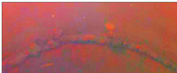
22. White water piping: Rust mounds on and beside a circumferential weld in another hot water pipe.
