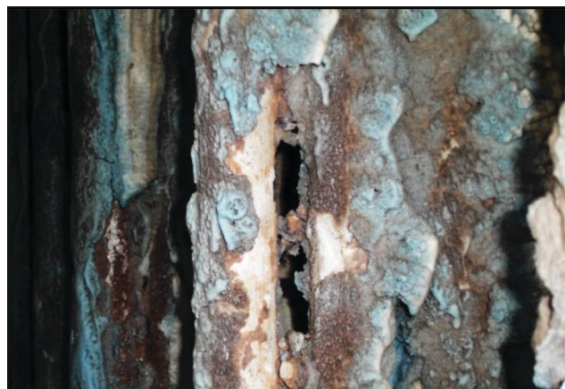
3. Blue deposits on secondary superheater platens in the recovery boiler at mill B.
