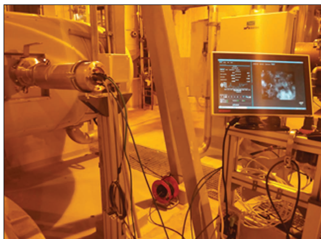
2. Bubble size measurement system installed in the process that includes on-site control and monitoring capabilities [4].
