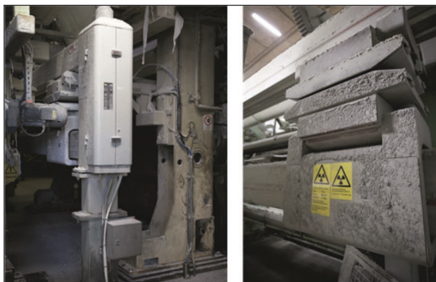
4. Onsite dust accumulation.
