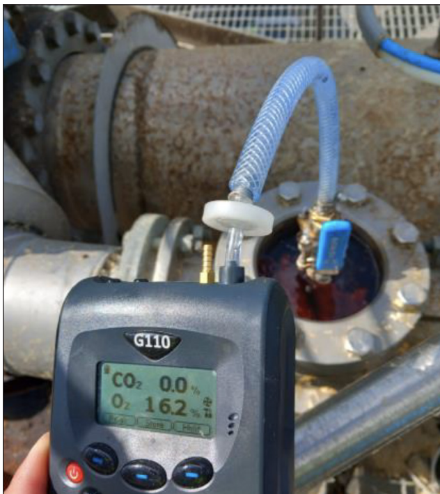
8. Sampling point and measurement for the residual gas in reactor 2.
