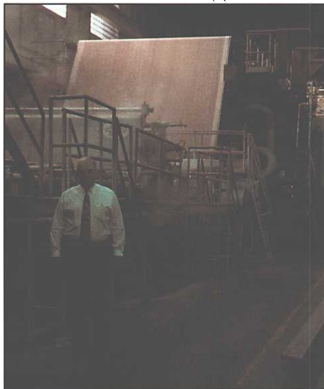
Mel Davidson and Rhinelander's rebuilt No. 7 paper machine
