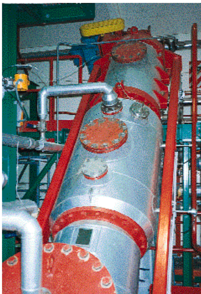
The fiber processing plant's liquor impregnation vessel
