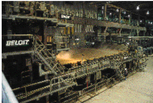
The forming section of the No. 2 linerboard machine
