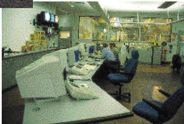
The control room
