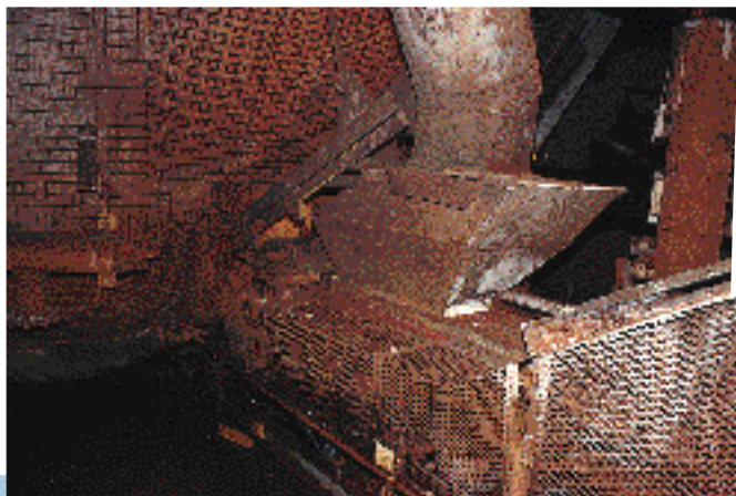
(top) Iron oxide addition point for the DARS furnace
