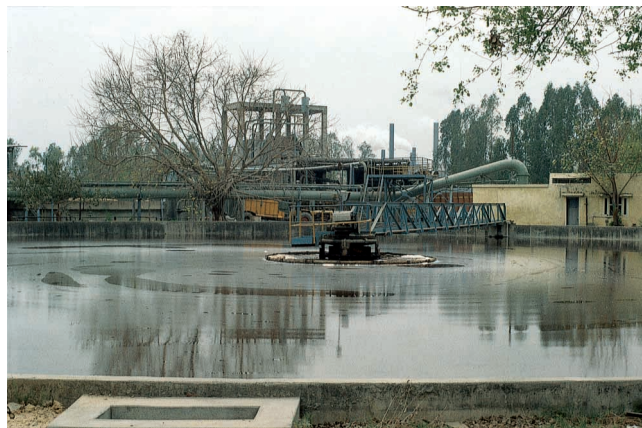
Shree Gopal's secondary clarifier for effluent treatment
