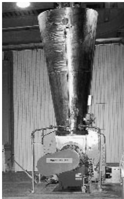
A tour of the mill included a stop at the refiner.
