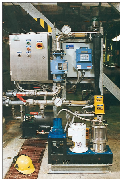
5. Paprispec ® prototype used in mill installation
