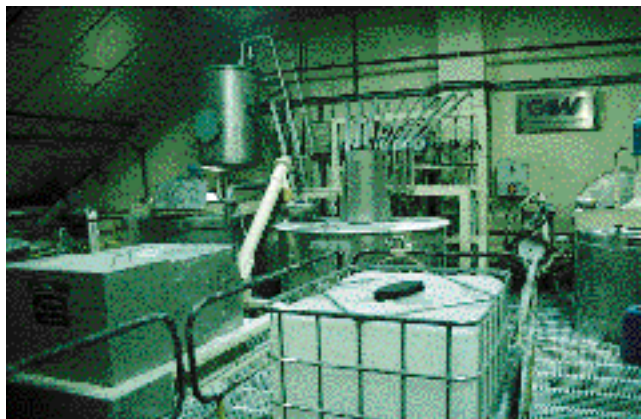
The mill has modernized its chemical storage and mixing area
