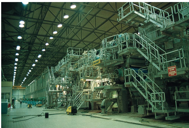
The Valmet machine and dryers
