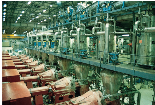
Siemens drives and Sunds refiners
