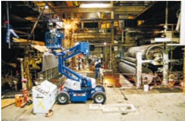
2. Size press area during shutdown, Jan. 20, 1998
