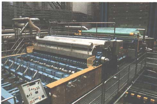
The beginning of the pulp finishing line
