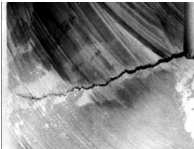
25. Crack in head spigot
