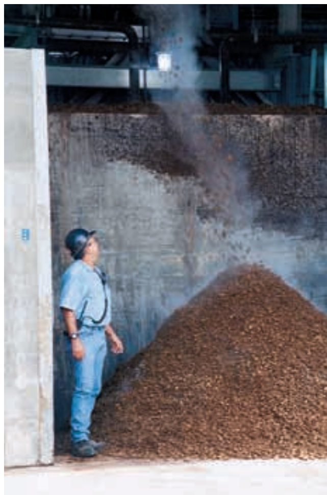
Press cake drops to a concrete bunker at ground level prior to being transported to the hog fuel boilers.
