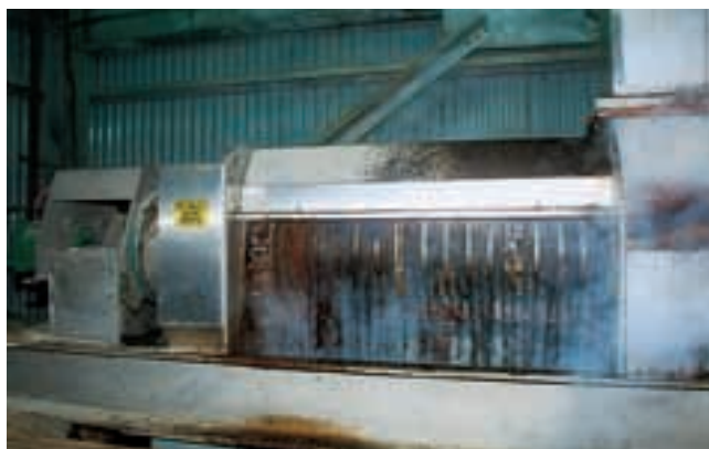
The flow of hot black liquor being squeezed from the quaternary rejects is seen dramatically when the screw press covers are removed.
