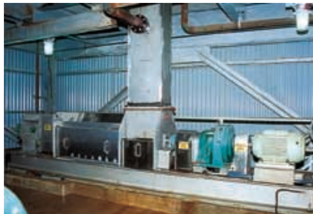
One of a pair of Vincent Model VP-12 presses. Tailings from sidehill screens on the floor above drop through the vertical chute into the press.
